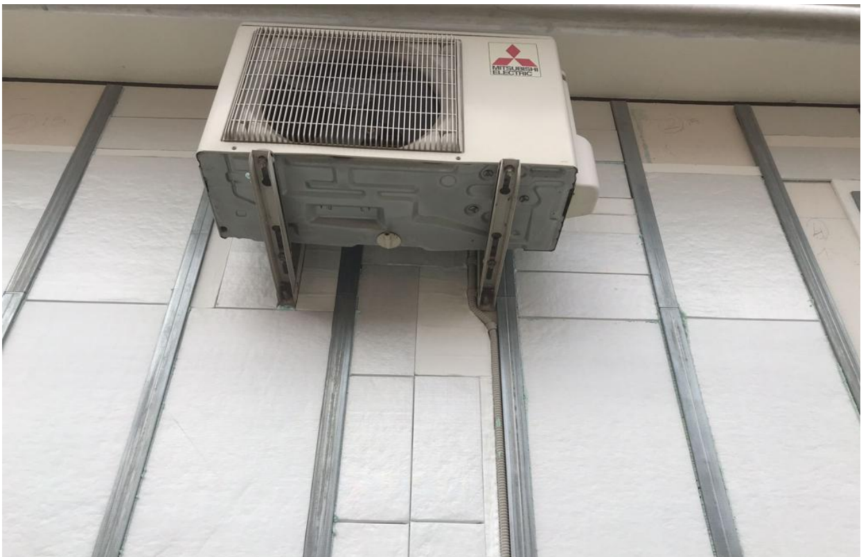
(CZ detail under air-conditioning machine)
