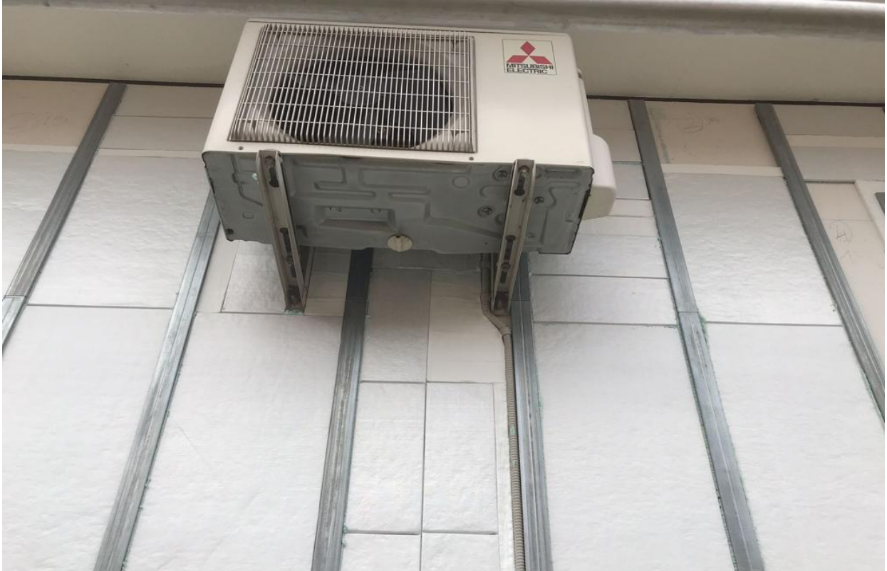
(CZ detail under air-conditioning machine)
